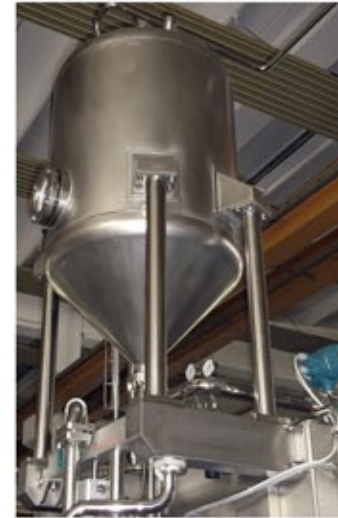
Aseptic storage tank (accessory) and electromagnetic flowmeter for the capacity measurement
