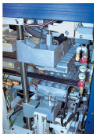
RDKP 72g forming station
